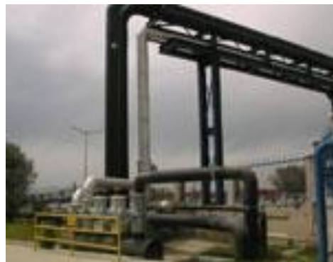
Figure 5.9: Example Pipe Bridge
